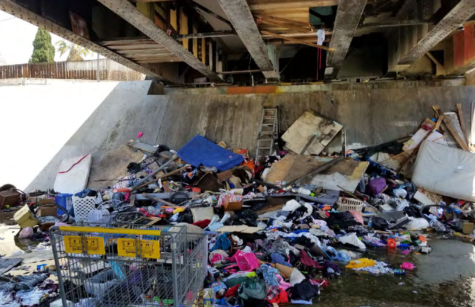
Figure 382. Large amounts of trash and debris are common conditions underneath bridges along the LA River. Source: LA County Public Works, 2018.
