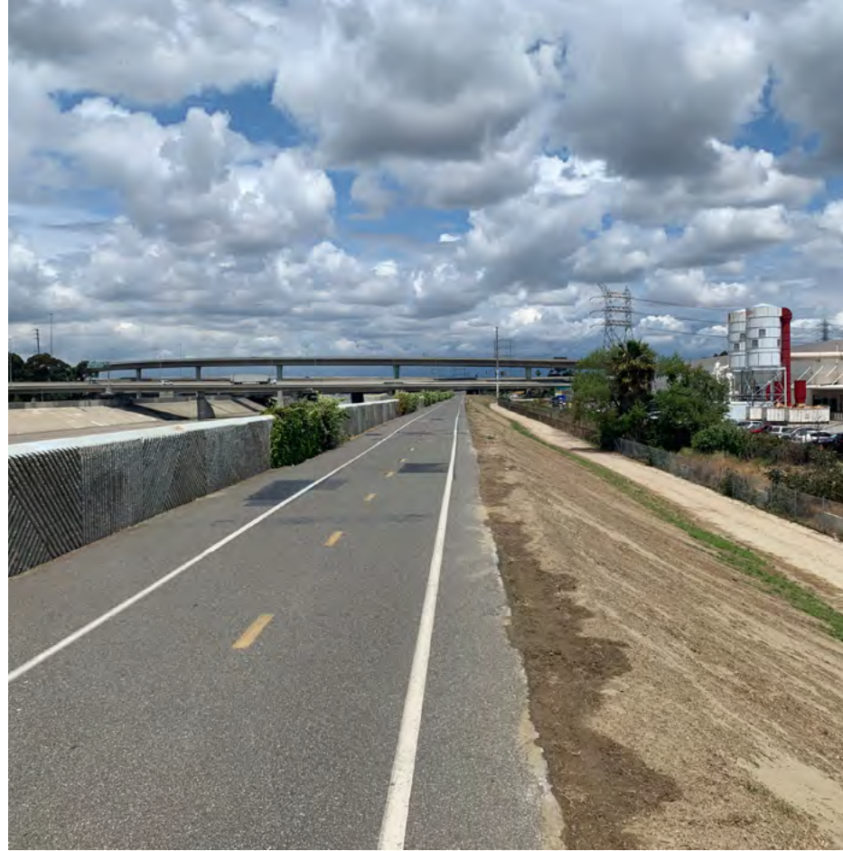
Figure 62. The lower river's parapet walls, such as these shown at river mile 10.1, were installed in the late 1990s in order to increase the channel capacity to greater than the 1% event. Source: OLIN, 2019.
