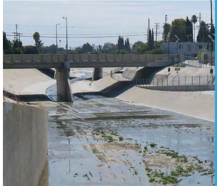
Figure 265. The existing trail dips below street level at the Mason Ave undercrossing near river mile 49.8. Source: OLIN, 2019.
