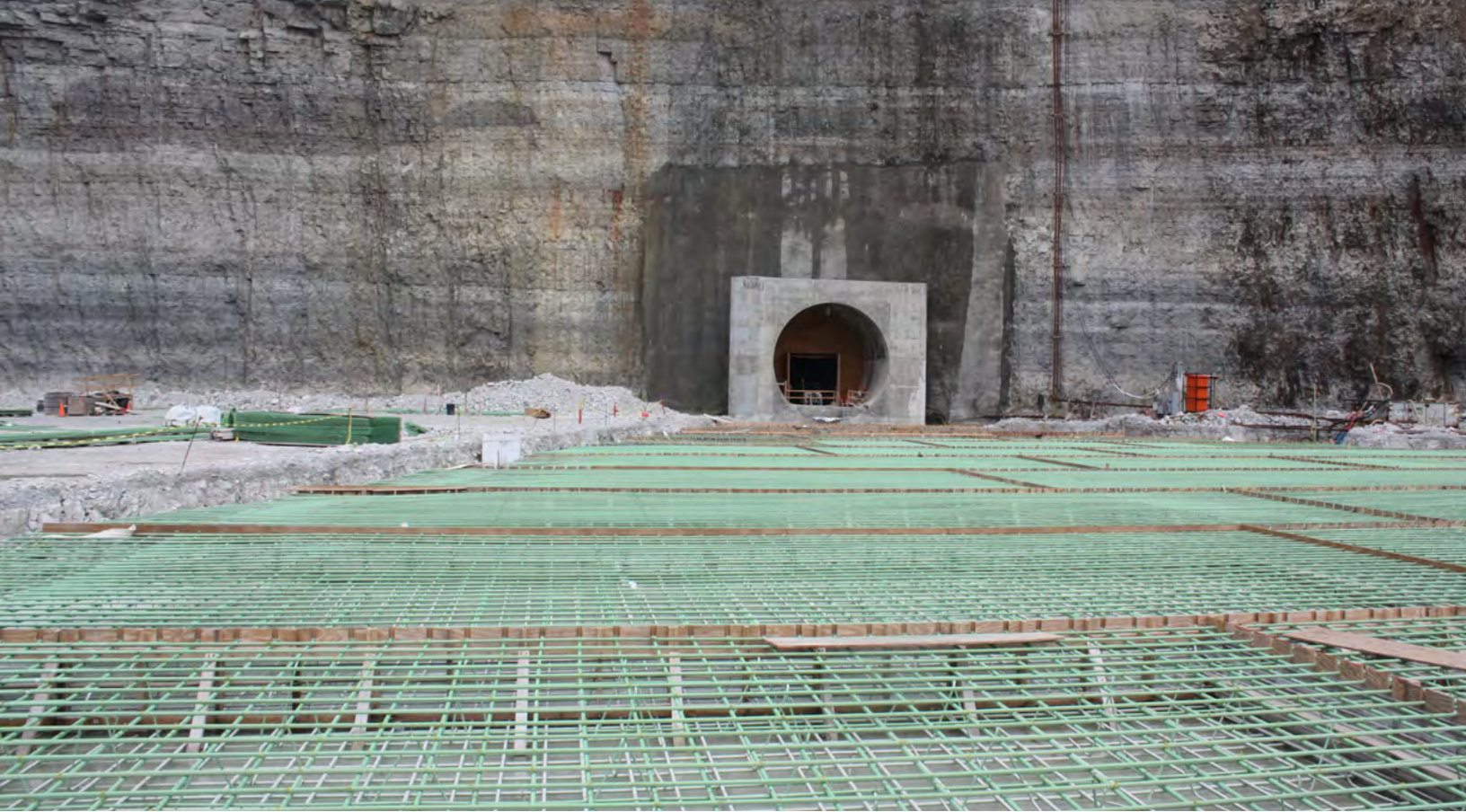
Figure 279. Excess rainfall and combined sewage overflow runs through a series of tunnels deep underneath Cook County in Illinois. The water discharges into large reservoirs where it is held until it can be treated and released back into the water system. Source: OLIN, 2019.
